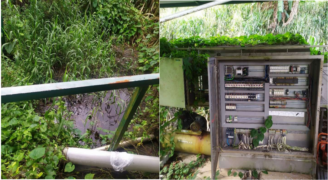
Figure 13. Septic tank with sewage and liquid waste and Figure 14. Faulty control panel responsible for the functioning of the water treatment plant
