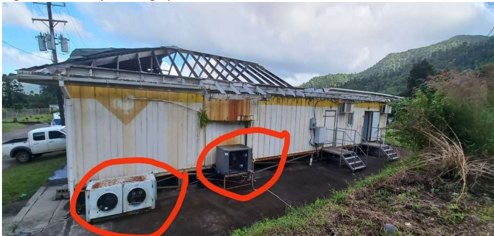
Figure 19. faulty cooling system
