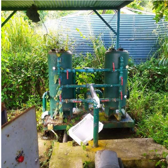
Figure 17. water purification tank
