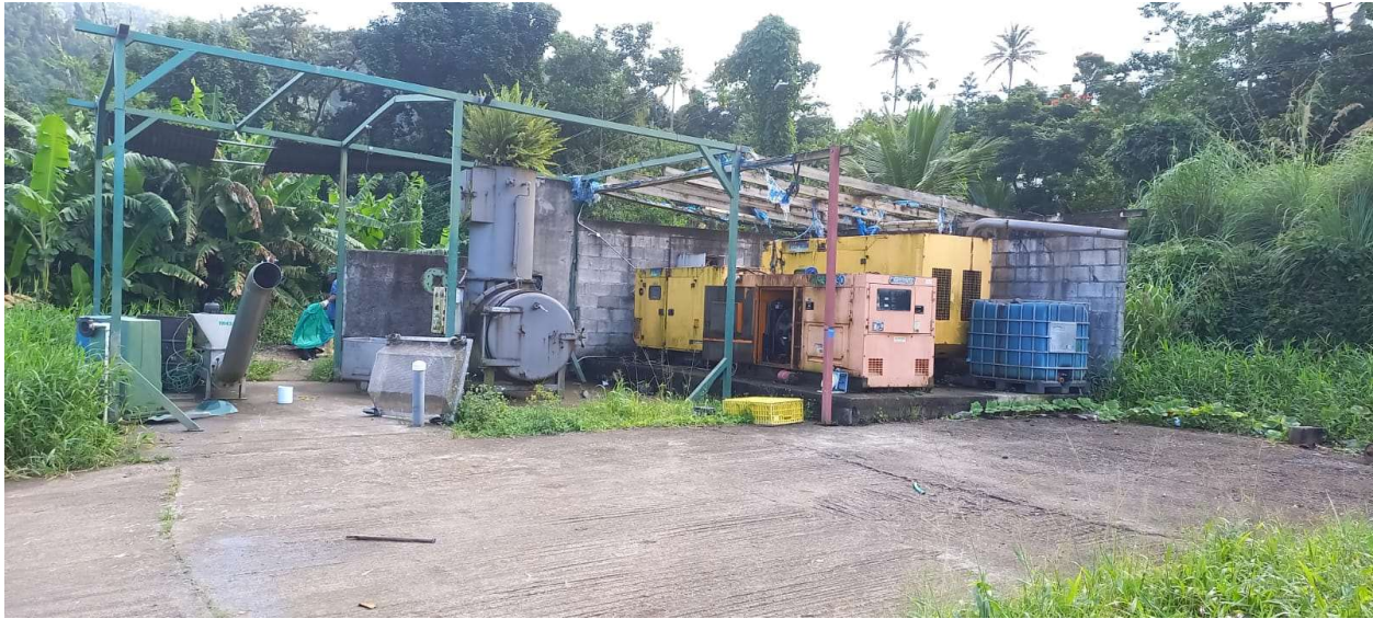
Figure 10. Incinerator and generator shed
