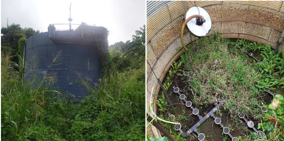
Figure 15. Sequencing batch reactor (SBR)(outside) Figure 16. SBR (inside)
