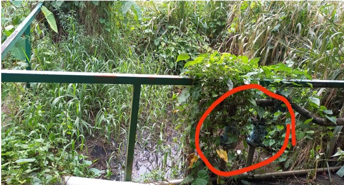
Figure 20. Pipes from homogenizing tank to the sequencing batch reactor (SBR)
