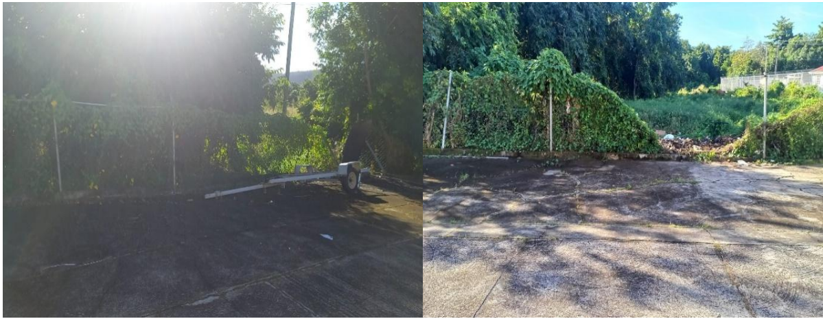
Photo 5. Windows to be installed with mesh Photo 6. Area for concrete pavement (Roseau)
