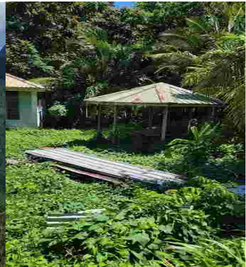
Photo #8. Gazebo at Ross Castle to be repaired
