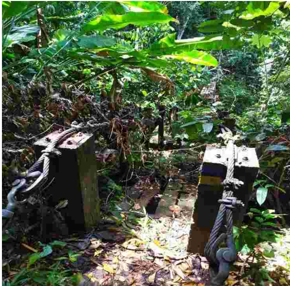
Photo # 9. spring bridge to be renovated
