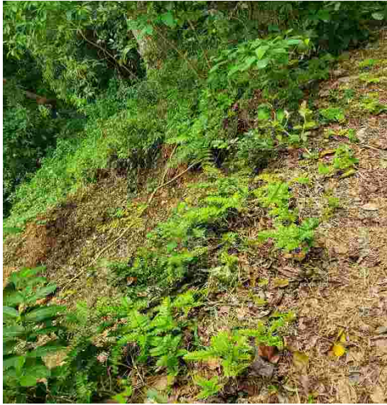
Photo # 12. Trail stabilization and expansion required
